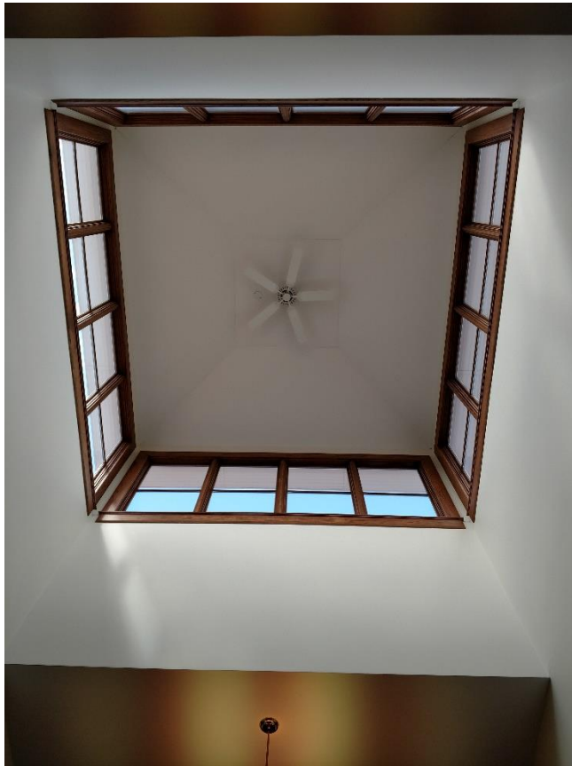
Looking upwards in the library's cupola, the fan in the above photograph will be removed before the artwork's installation.
